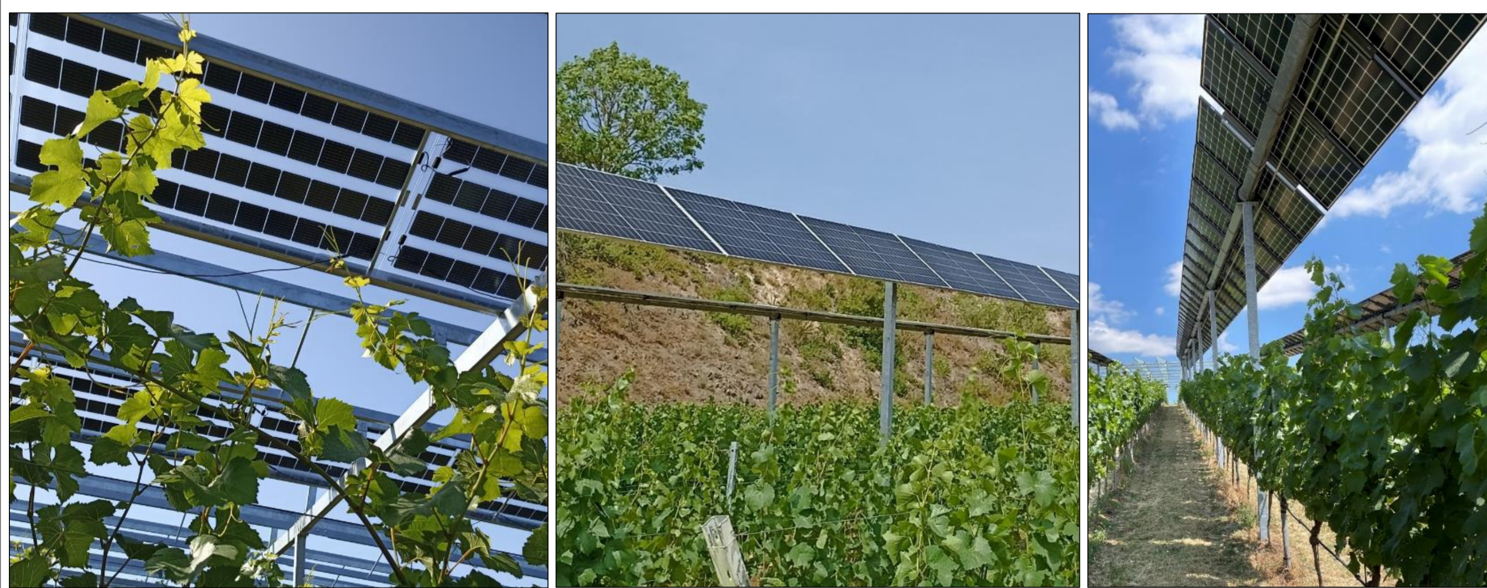
Fig. 1: Three different types of modules are installed at Blankenhornsberg: semi-transparent (left), single-axis tracking longitudinal (middle) and single-axis tracking transverse (right)
